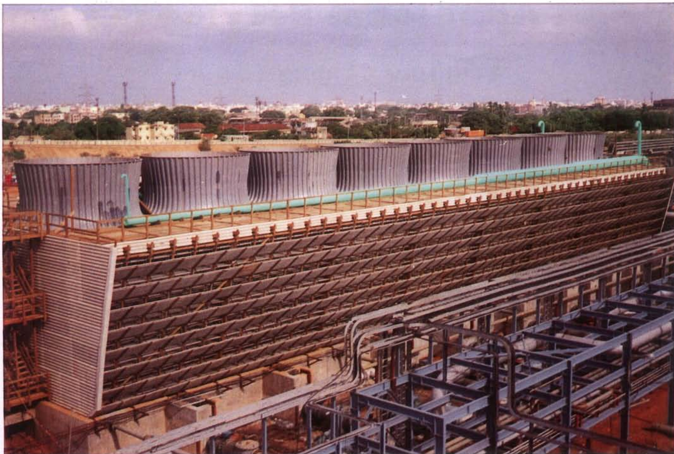
A Paharpur Class 500 Cooling Tower Model 586-6V-8, Serial No.97-2I-005, at GMR Vasavi Power Corp., Madras / 200 MW Diesel Power Station. EPC contractor – Hyundai Heavy Industries Co. Ltd., S. Korea.
